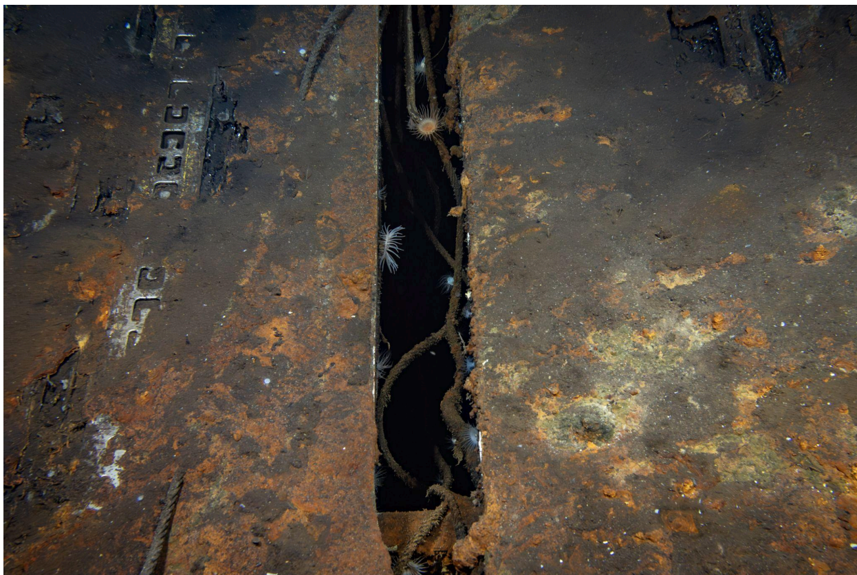
An expansion joint can be seen in the flight deck of Yorktown .
