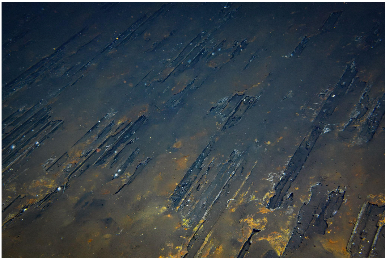
Condition of the wooden flight deck on board Yorktown .
