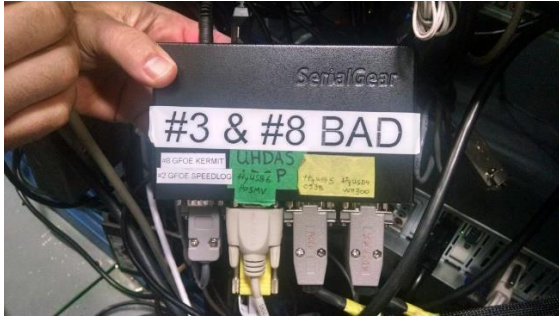
Figure 5. 8 port serial box behind the UHDAS machine
