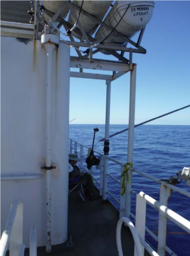
Stbd Aft: This station is mounted fwd of the stairwell on the 02 deck, as shown.
